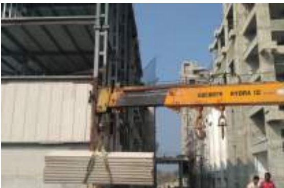
Fig 3 Aerated autoclaved concrete wall & block construction at MMRDA rental housing, Mumbai (Source: Aerocon, 2016)
