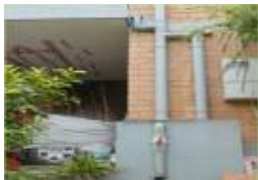
Fig. 15. Provision of Rain Water Harvesting Filter
